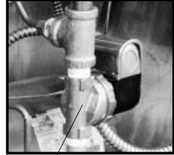
Typical cooling solenoid valve on RK units
